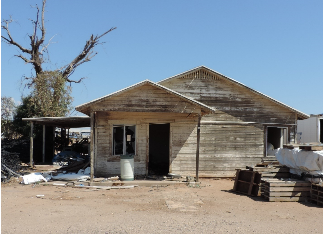
Photo 14. South elevation of worker house in the Central Village. View facing north. (Karen Krause photo, August 2023)
