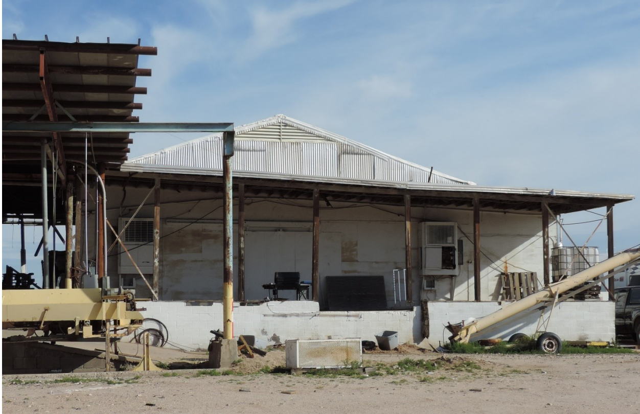
Photo 11. South elevation of the cold storage building as viewed facing north. (Karen Krause photo, August 2023)
