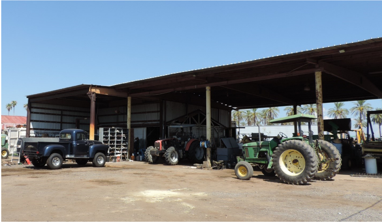
Photo 15. South and east elevations of the equipment shed as viewed facing northwest. (Karen Krause photo, August 2023)
