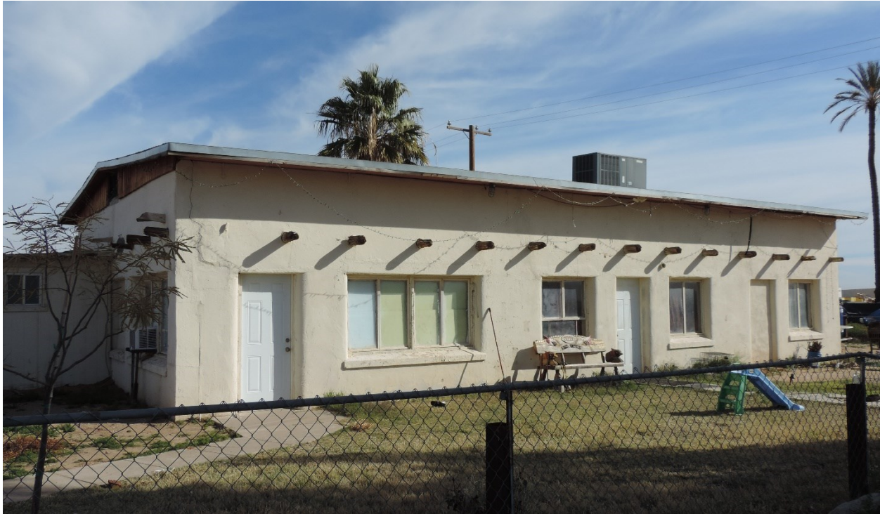
Photo 13. South and west elevations of the Ranch Office as viewed facing northeast. (Karen Krause photo, March 2023)
